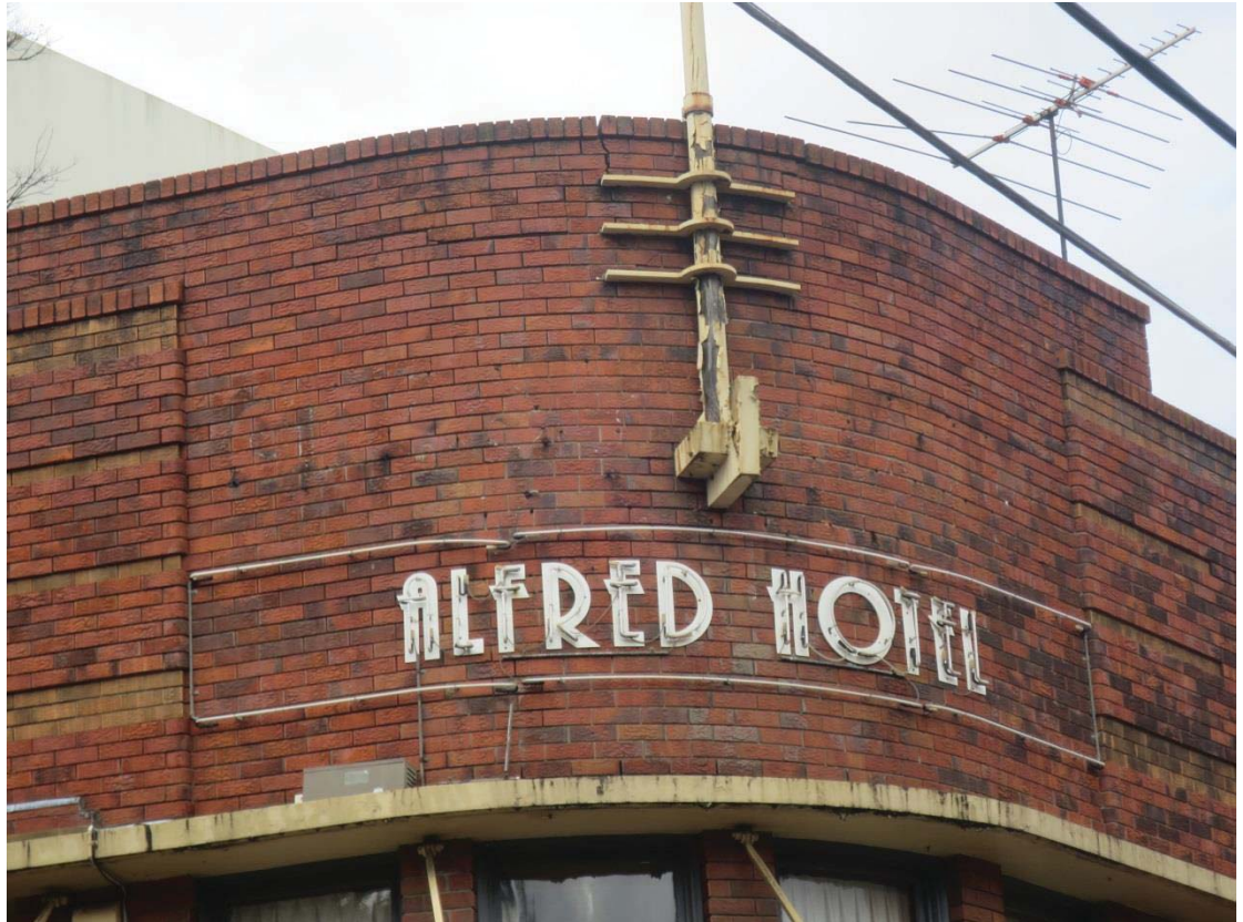
Figure 6 — cracks in the parapet are likely caused by rusting steel fixings attaching the flagpole.
