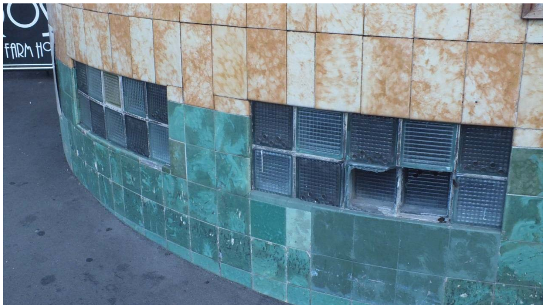
Figure 7 — damaged glass blocks lighting the basement near the street corner.
