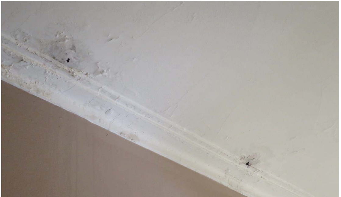
Figure 11 — view of water damage to ceiling at the western end of the first floor hall.
