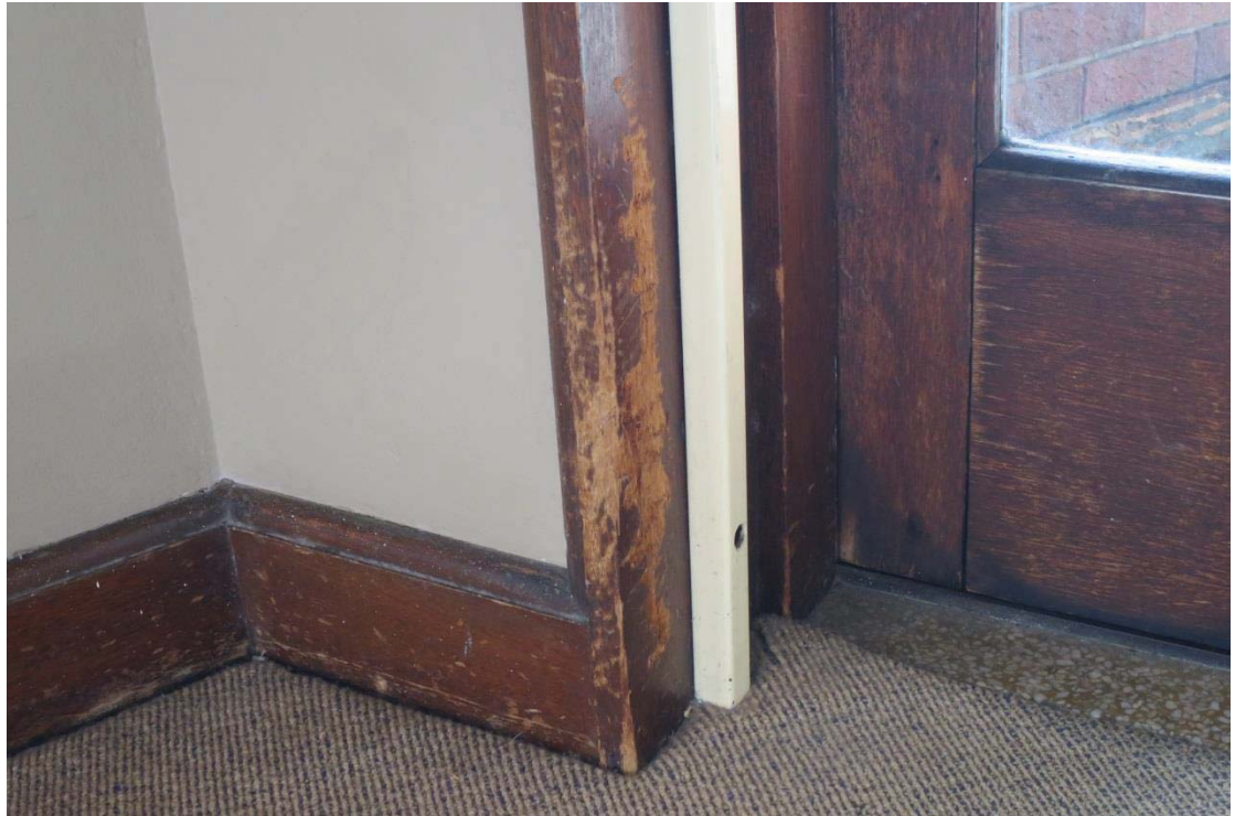
Figure 12 — impact damage to a simple section of meranti joinery in the first floor bedroom with a curved corner. Joinery elements with this degree of damage should be replaced to match.
